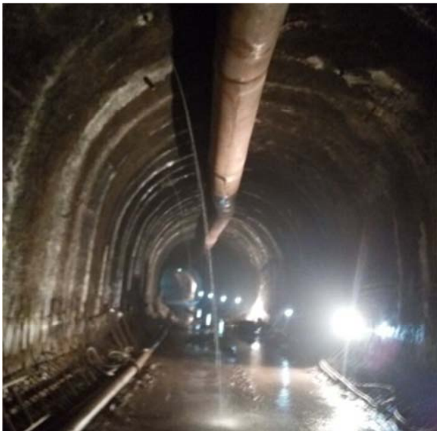
Figure 1. Photo of groundwater seepage in a tunnel.
